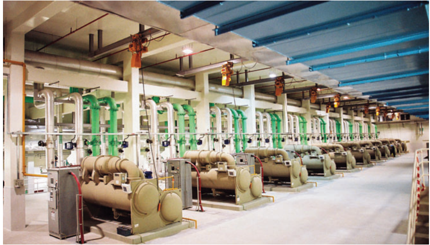
McQuay chillers in central plant
