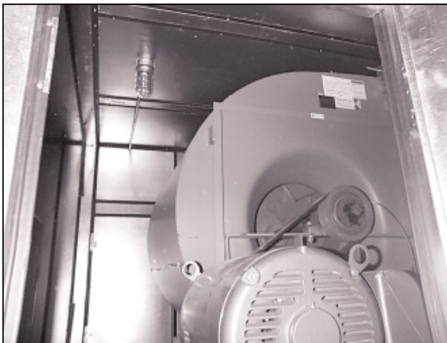
The Vision air handlers were shipped in sections, to overcome space limitations.
