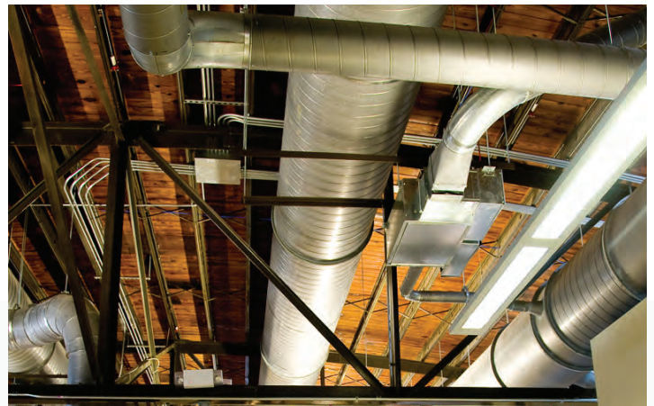
Southern Air's 3D Ductwork Modeling Software Enabled Best Use of Space in the Building's Existing Truss System
