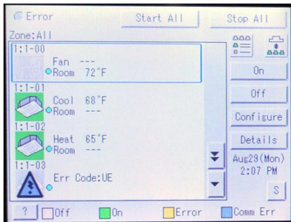
Figure 21, MicroTech III Air Handler Unit in Unoccupied Mode
