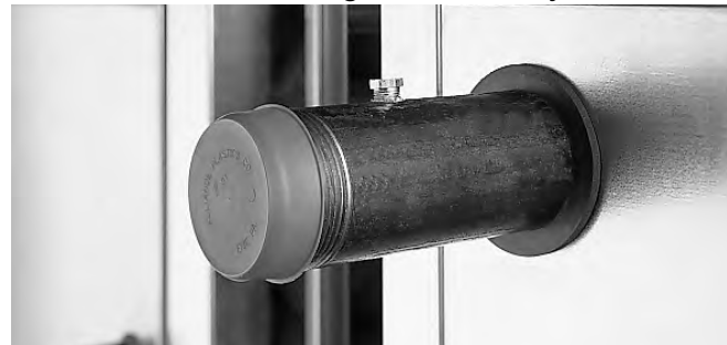
Figure 10: Coil Connections, Vents, Drains, and Drain Pan Connection, Extend Through Unit Cabinetry
