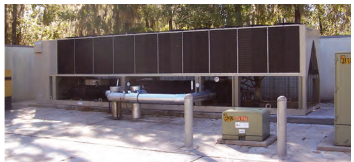
The 280-ton Pathfinder chiller with variable frequency drive provided improved efficiency and reliability.
